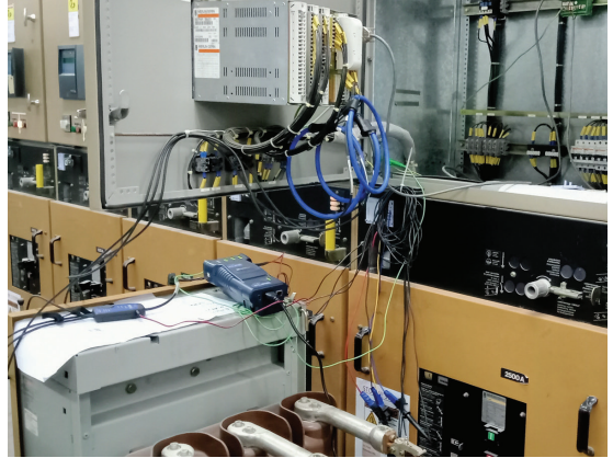
Power Quality Analysis Service for an 11kV Switchgear
