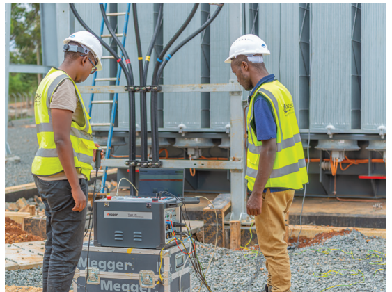
55 MVA Power Transformer Test
