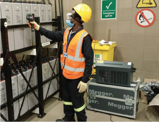
Battery Testing at Bujagali Energy Limited, Uganda
