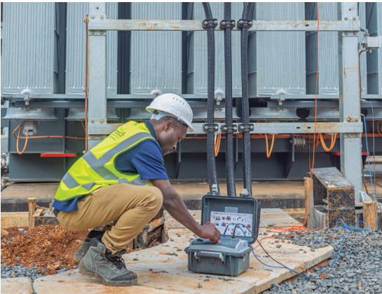
Insulation Test on a Power Transformer
